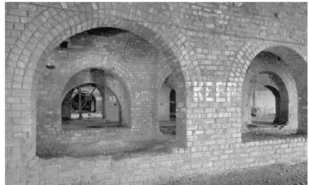
Figure 4.8: Lady Victoria Colliery, 1999. View beneath the picking tables showing the arcades of brick arches separating the railway sidings which passed under the colliery. SC894274
